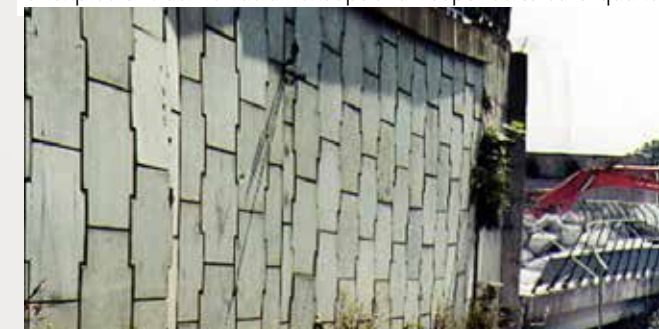
After the Izmit earthquake in 1999 - Turkey
