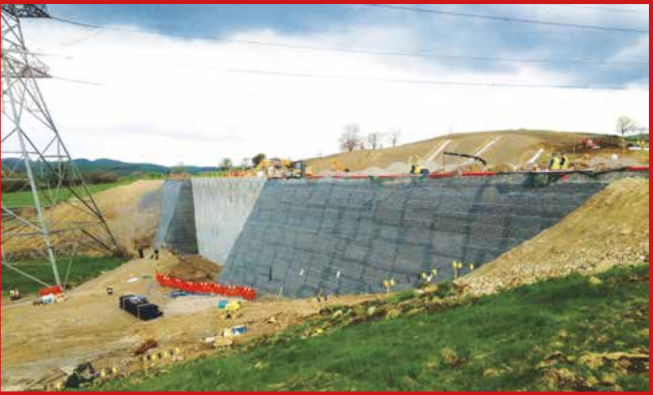
Cumbria Electric sub-station - Old Hutton, UK
