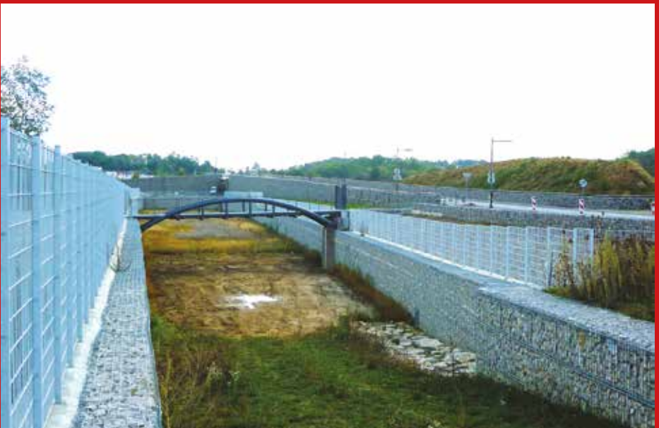
Storm water basin - Decines, France
