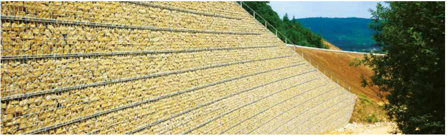
Road RD31 - Dortan, France
